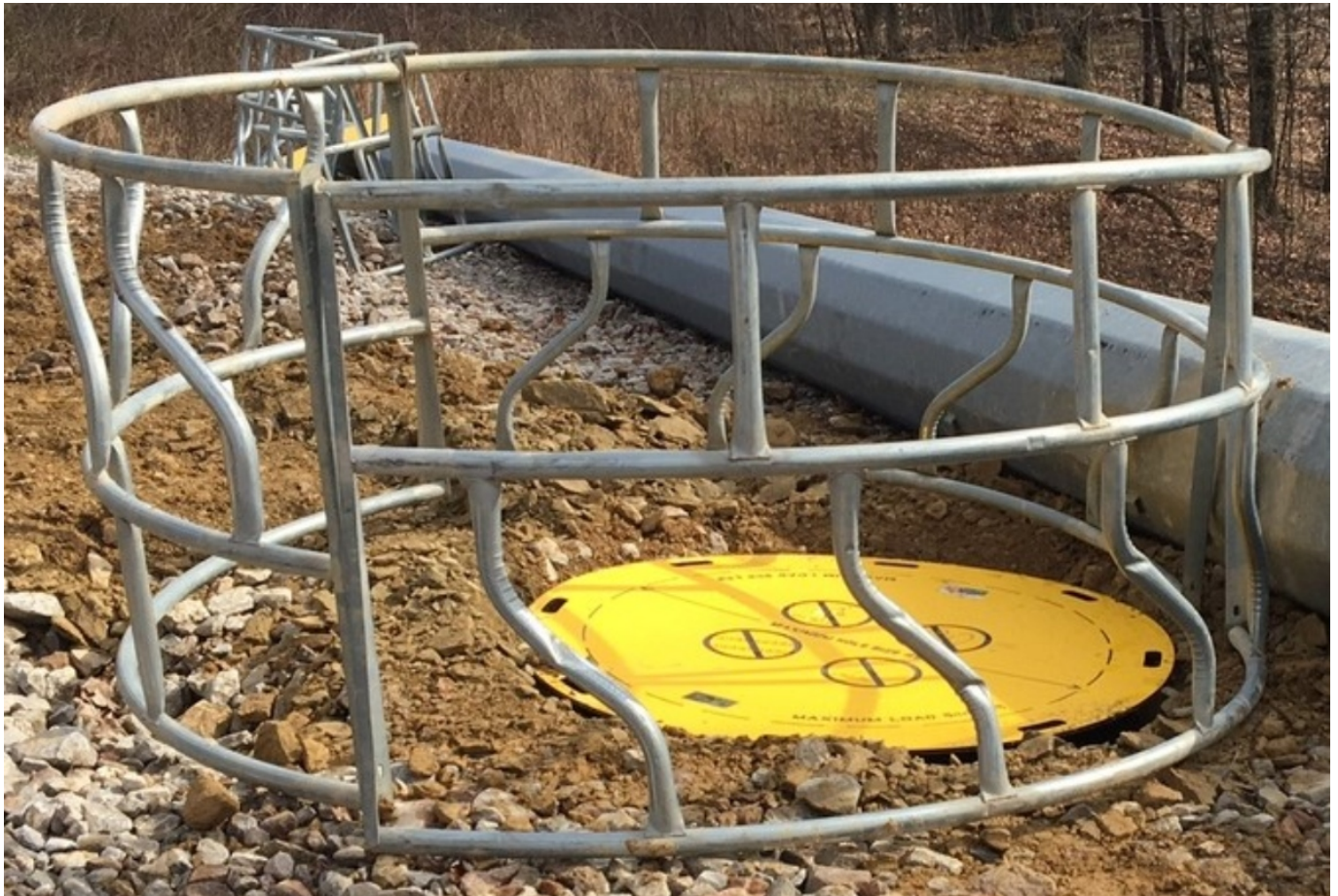
Pole Hole Cover in use
